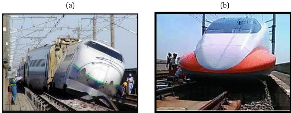
Fig. 4. Seismic effects on High Speed Railway & its structures (a) Derailment of high-speed trains on bridges due to Niigata Chuetsu earthquake (b) Derailment of high-speed trains on bridges due to Taiwan earthquake
